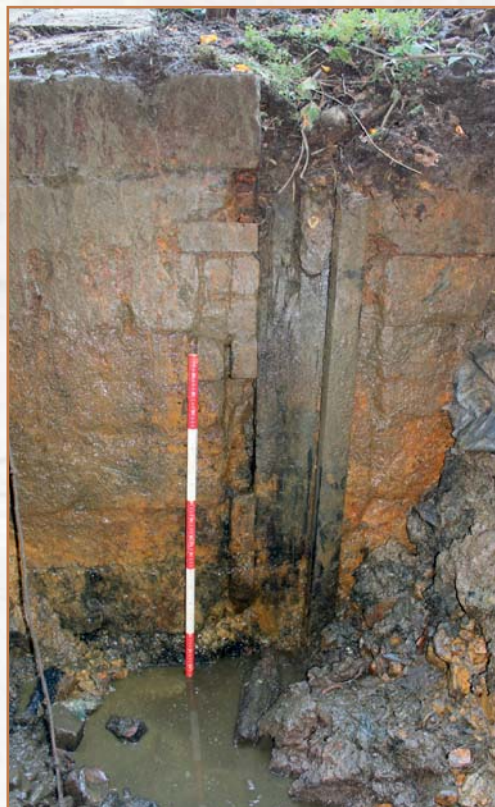
The vertical slot set into the stone revetment wall of The Island
