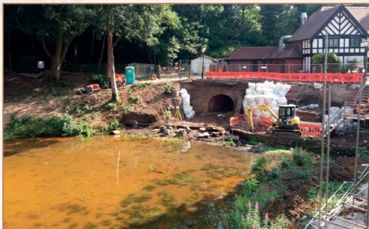
The tunnel and the small quay that were uncovered during the restoration works in 2018, showing the half-timbered building that replaced the corn mill in the early 20th century
