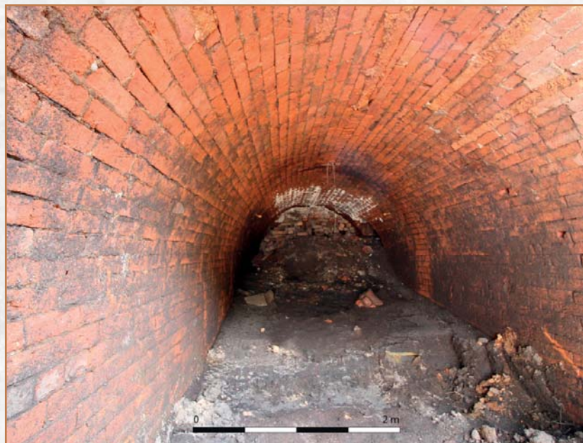
Interior of the tunnel between Worsley Delph and the former corn mill
