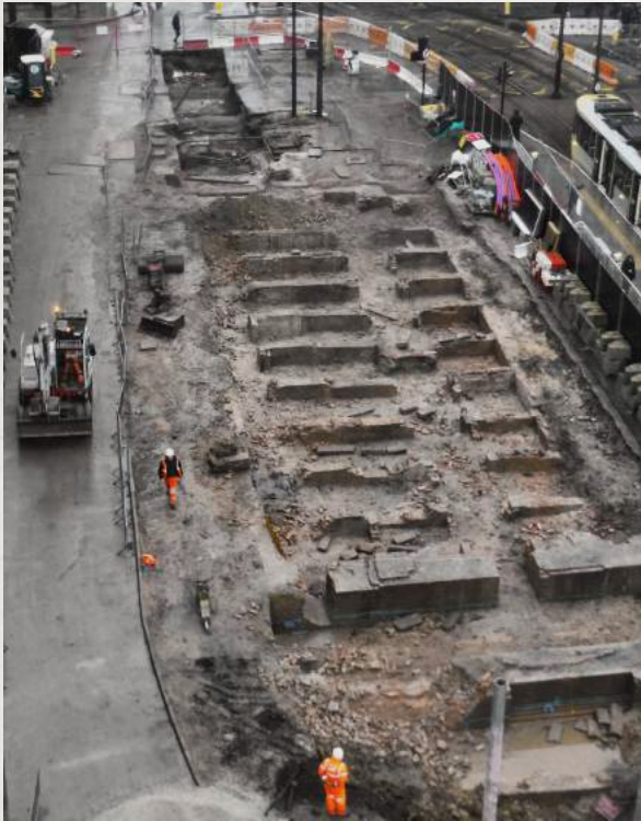
Aerial view of the foundations and crypt of St Peter's Church during the excavation
