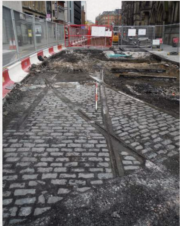
Old tramlines exposed at the junction of Princess Street and Albert Square, in front of Manchester Town Hall
