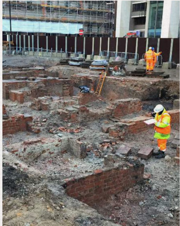
The exposed foundations and crypt being recorded by archaeologists during the excavation
